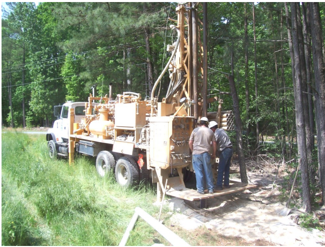
North Carolina Division of Water Quality drilling rig installing regolith groundwater observation well in southern Orange County during 2011.
