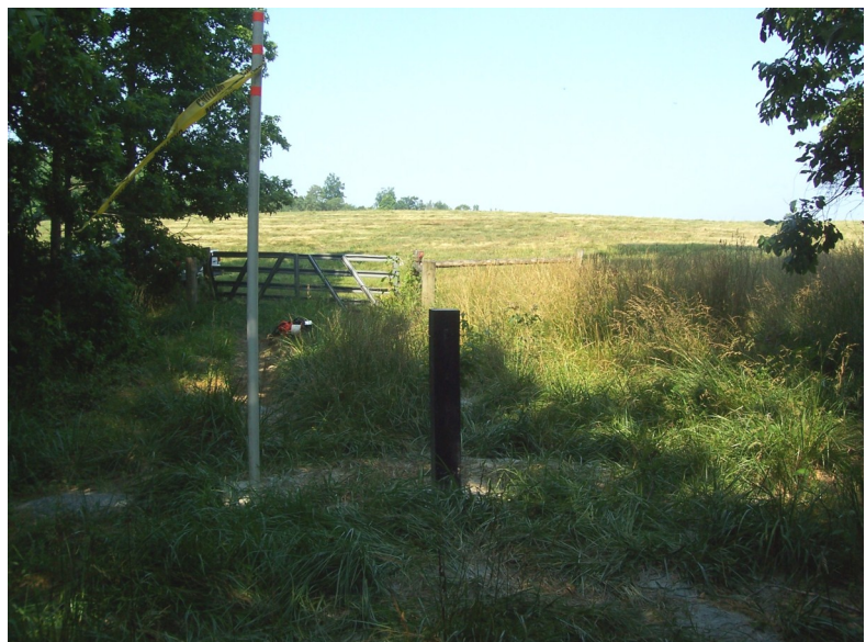
Regolith groundwater observation well installed in 2011 in southern Orange County.
