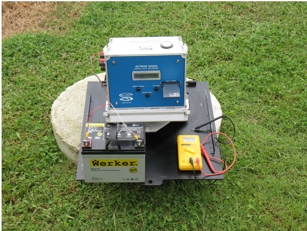
Sutron including card reader, 12-volt battery and voltage meter
