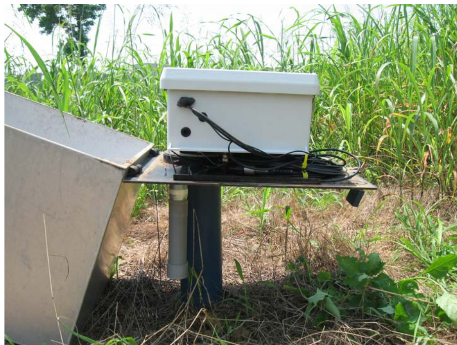
Solinst Telemetry System. Cell phone antenna is housed in a PVC pipe projecting downward from shelter base.
