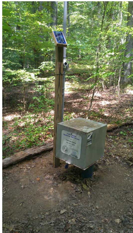
STS Final Installation Complete with Solar Panel
