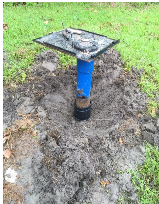
Corroded Well Casing in Need of Repair, East Lake Station, J7K, Dare County
