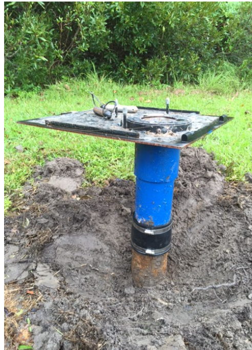
Well Casing Repaired Using Flexible Rubber Boot, East Lake Station, J7K Dare County
