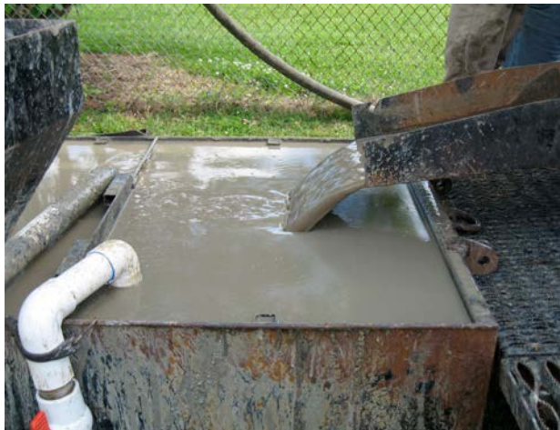
Mud Rotary Drilling using Mud Circulation Tank Farmville Station, M 27U, Pitt County
