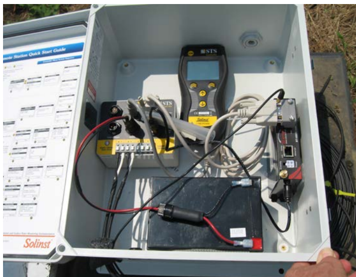
STS Equipment Lewiston Station, H 22I, Bertie County
